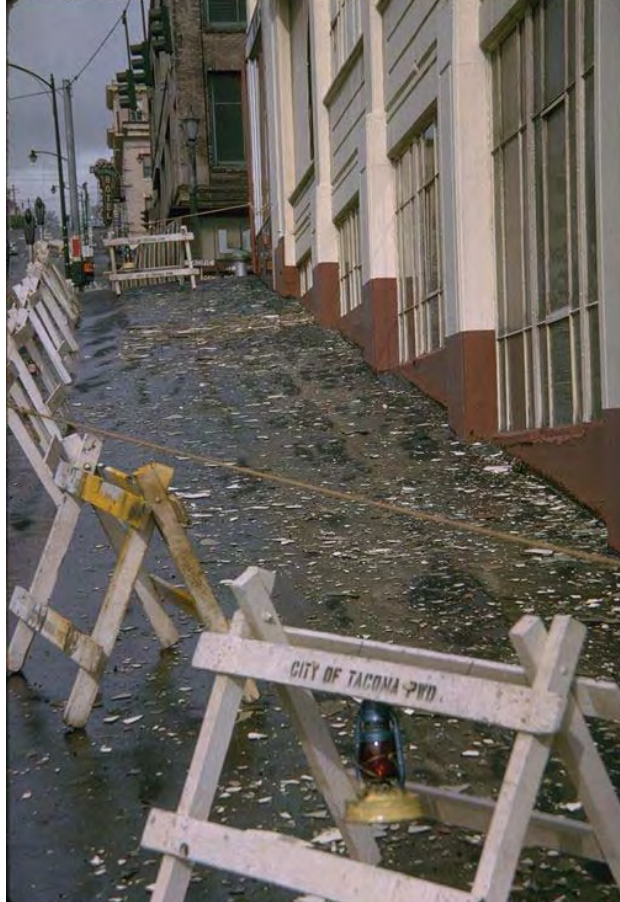
Figure 1.2 Damage to window systems observed during the Puget Sound, Washington, 1965 earthquake. (Courtesy of the National Information Service for Earthquake Engineering, EERC, University of California, Berkeley)
