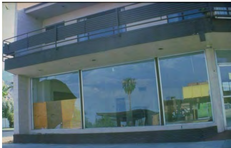
Figure 1.1 Damage to window systems observed during the Palm springs, 1986 earthquake. (Courtesy of the National Information Service for Earthquake Engineering, EERC, University of California, Berkeley)
